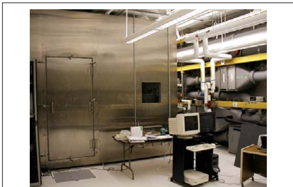
Figure 1. Building Energy and Environmental Systems Laboratory at Syracuse University.
